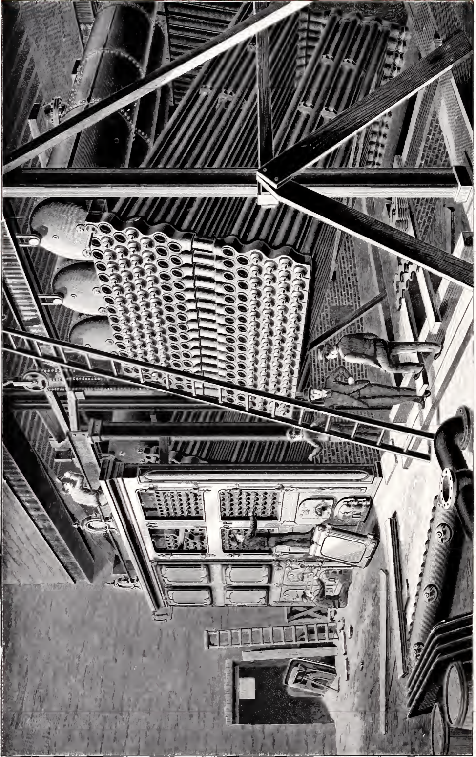
"Double-deck" Babcock & Wilcox Boilers at Cleveland City Cable Railway Co.'s, Cleveland, O., 1,086 H. P. Erected 1890.
